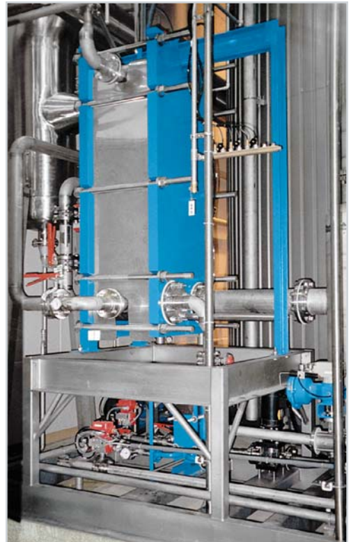
An Accu-Therm used in a heating and cooling system.
