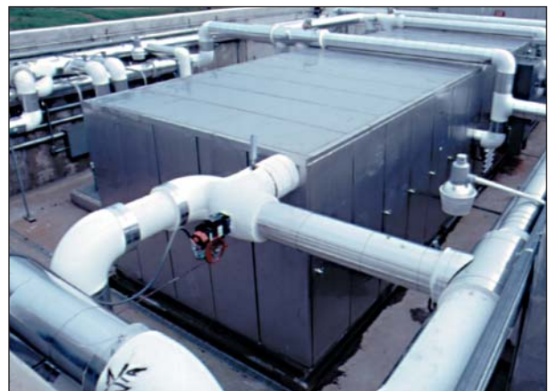
Two 150-TR units installed at a northeastern electric utility's administration building.
