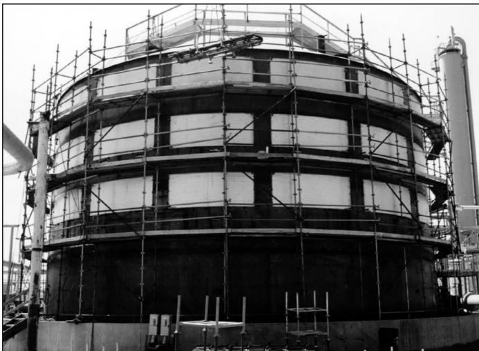
Installation of Mueller Temp-Plate double-embossed clamp-on sections at a large oil refinery.
